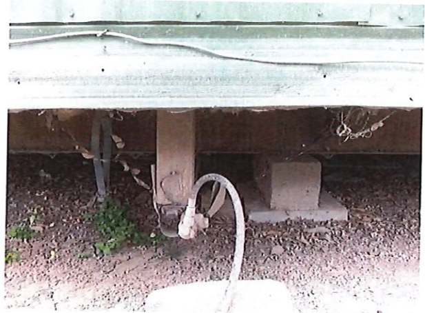
propane tank connection and footing
