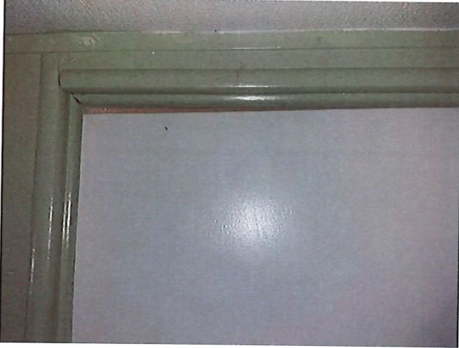
Bathroom door does Not close properly
