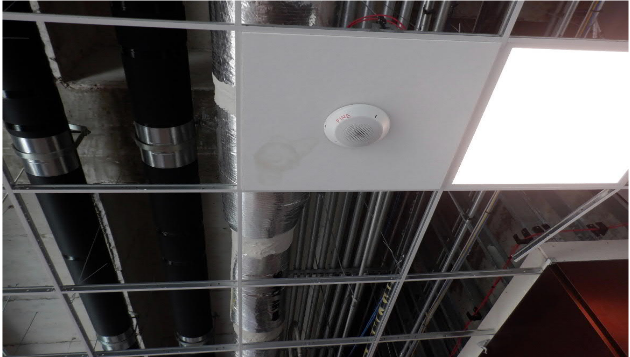
Photo #9 View of moisture stains on ceiling tile in the western area of the 7 th Floor Public Circulation 7A-001.
