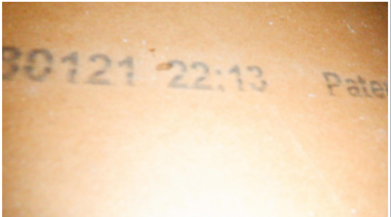
Photo #12 View of wall cavity for Photo #6 location. No moisture stains/fungal growth observed.
