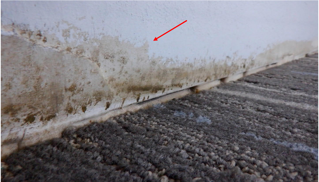
Photo #5 View of moisture impacted lower gypsum wallboard observed in the north portion of the 2 nd Floor Justice 4, 2B-134. No fungal growth reported in surface sample TL-2.
