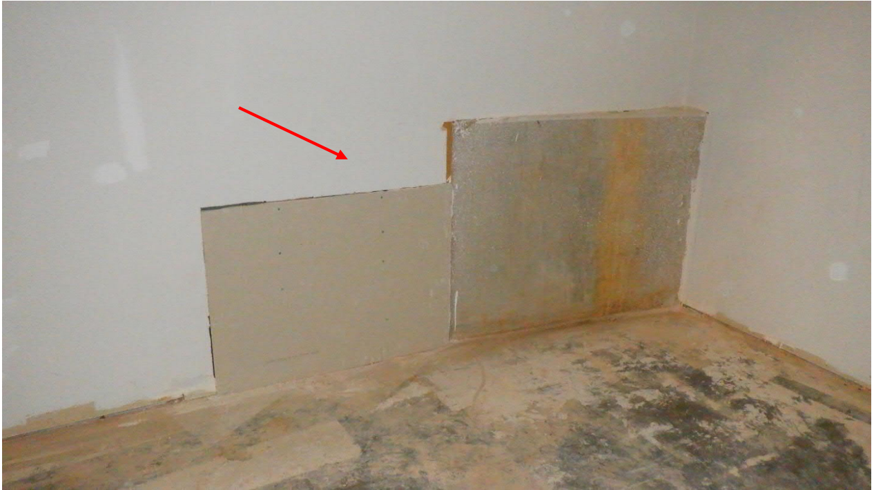
Photo #3 View of area where moisture/fungal impacted gypsum wallboard was removed and replaced in the southeast portion of the 1 st Floor Stair No.1 ST-1A1.
