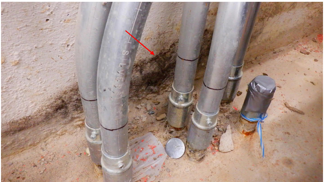
Photo #2 Closer view of fungal growth locations observed on northwest lower CMU block/concrete wall in 1 st Floor Electrical Room 1A-158.
