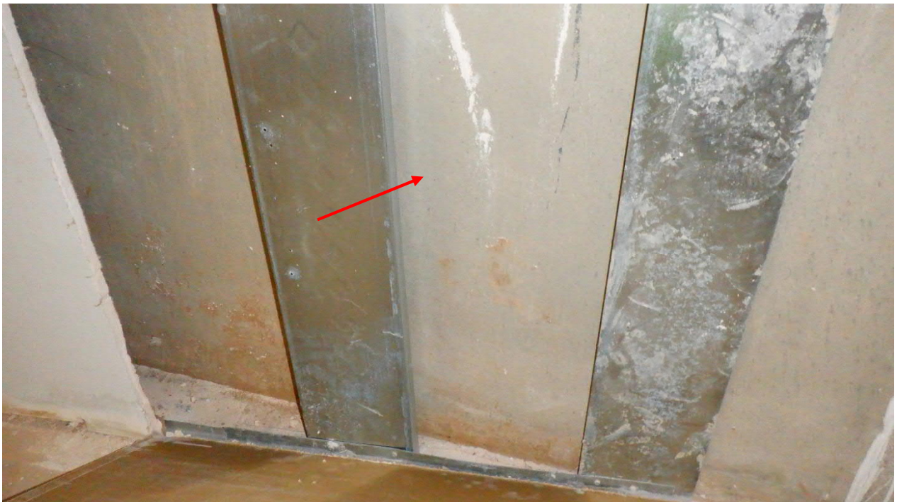
Photo #4 View of wall cavity for Photo #3 location. No moisture stains/fungal growth observed.
