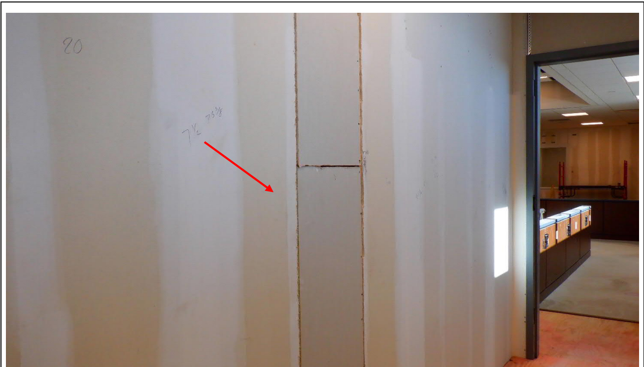
Photo #11 View of area where moisture/fungal impacted gypsum wallboard was removed and replaced, west wall of Entrance to 7 th Floor Courtroom 7B-600.
