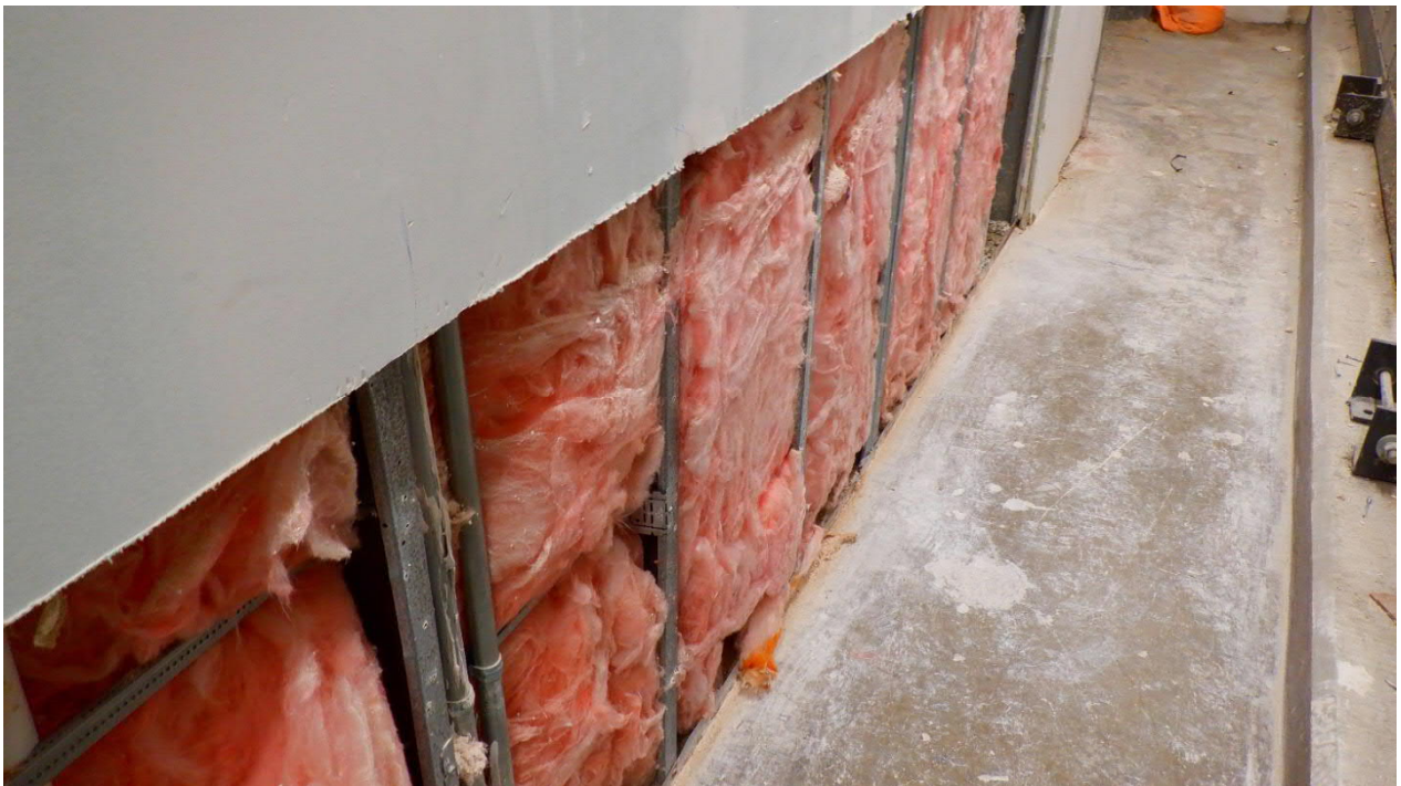
Photo #6 View of area where moisture impacted gypsum wallboard was removed in the east portion of the 2 nd Floor Electrical 2A-146 and Mechanical 2A-147.
