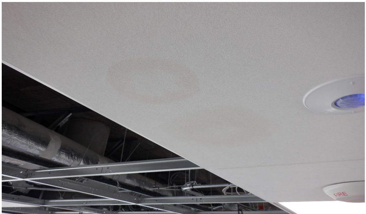
Photo #10 View of moisture stains on ceiling tile in the center area of the 7 th Floor Public Circulation 7A-001.
