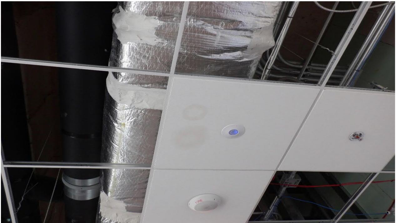
Photo #8 View of moisture stains on ceiling tile in the center area of the 3 rd Floor Public Circulation 3A-001.
