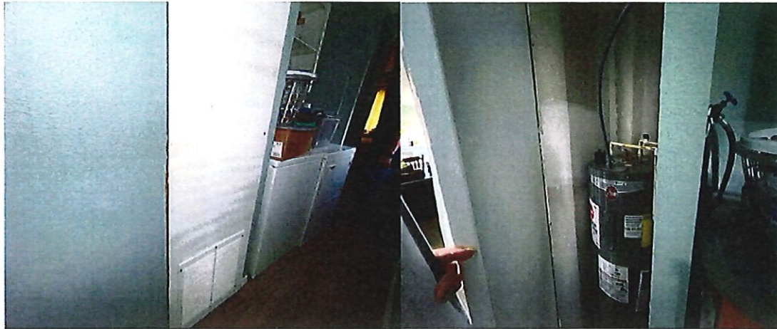
Laundry area and home boiler
