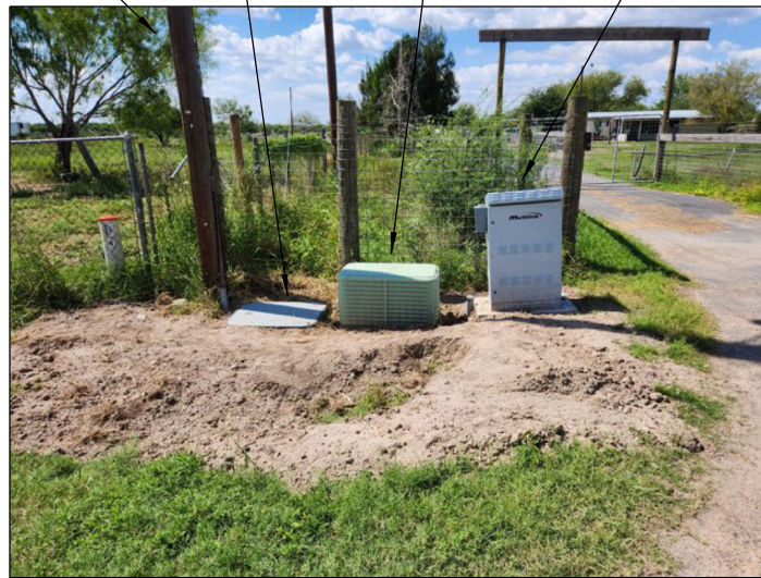
LAT: 26.330874 LONG: -98.058222 NEW SPECTRUM UG POWER SUPPLY 3' IN ROW & 14.5' FROM EOP
