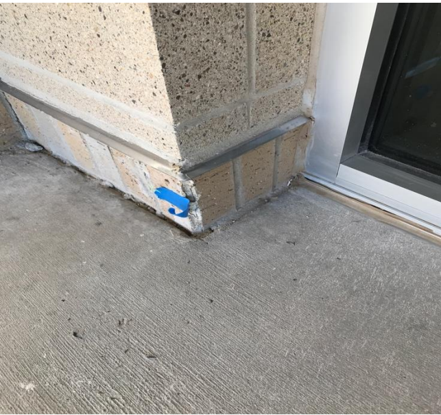
Brick is broken in from entrance
