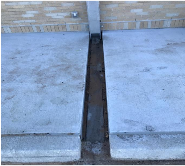
Both metal grates missing
