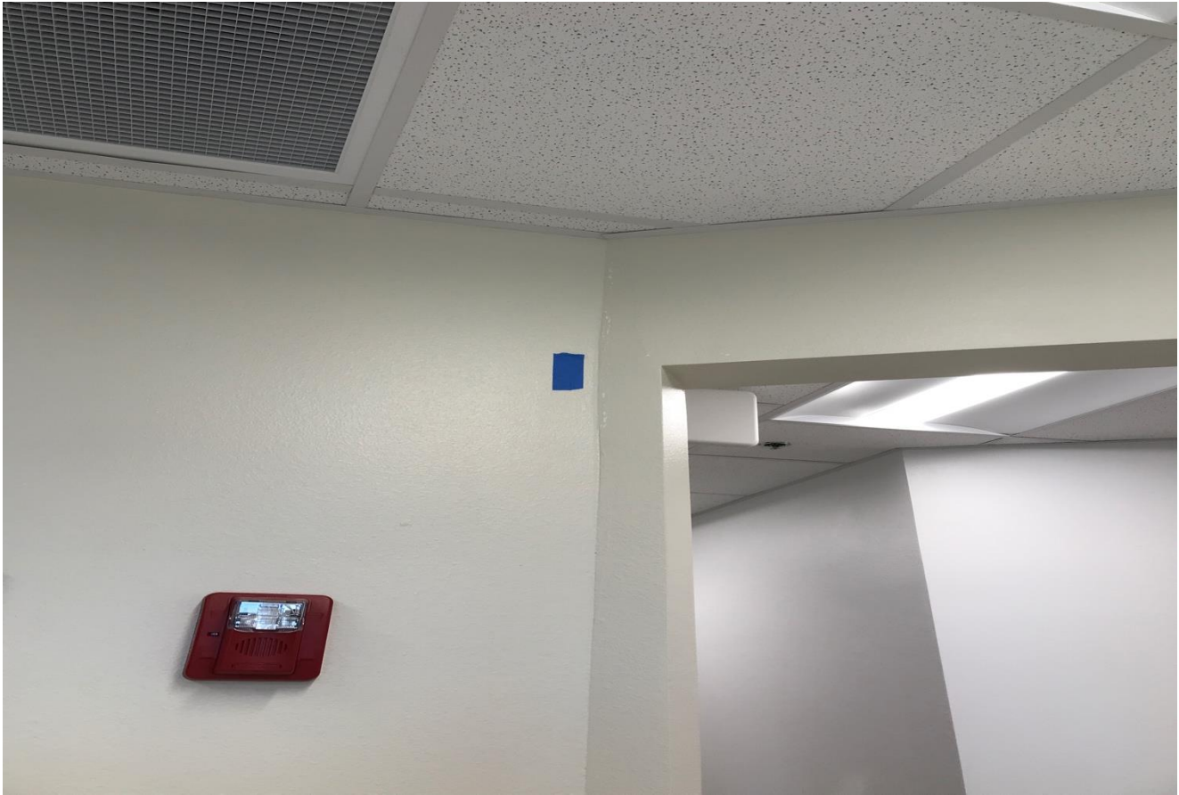
Paint touch up needed above case opening in receptionist area
