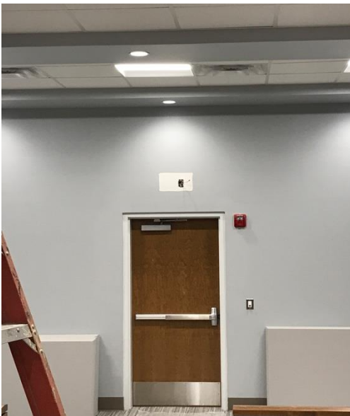
A104 exit sign missing from above door
