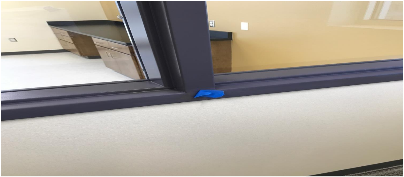
Rm A114 frame needs to be sanded and repainted
