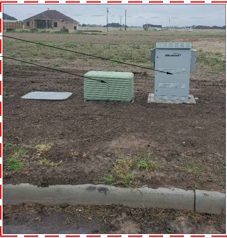
LAT: 26.214585° - LONG: -98.001431° NEW SPECTRUM UNDERGROUND POWER SUPPLY 2' NORTH FROM ROW & 5' SOUTH FROM EOP
