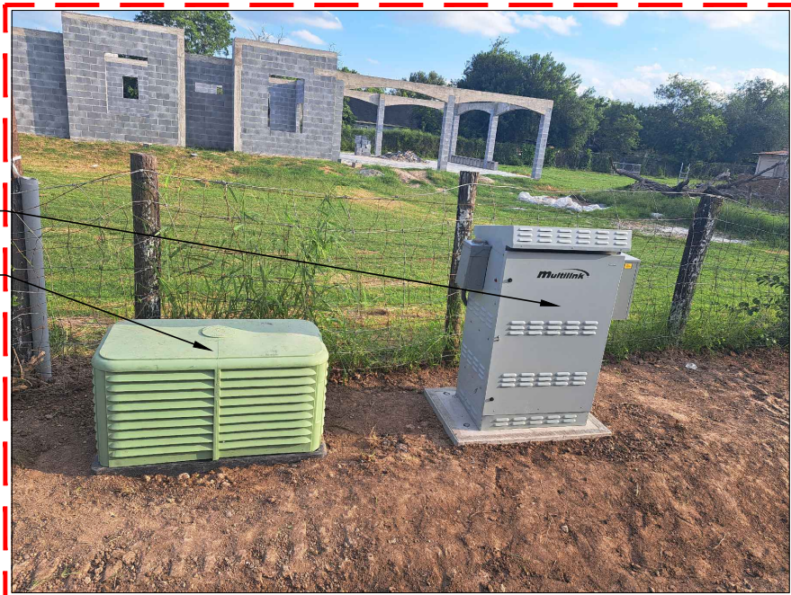
LAT: 26.238622° - LONG: -98.011589° NEW SPECTRUM UNDERGROUND POWER SUPPLY 1' NORTH FROM ROW & 10' SOUTH FROM EOP
