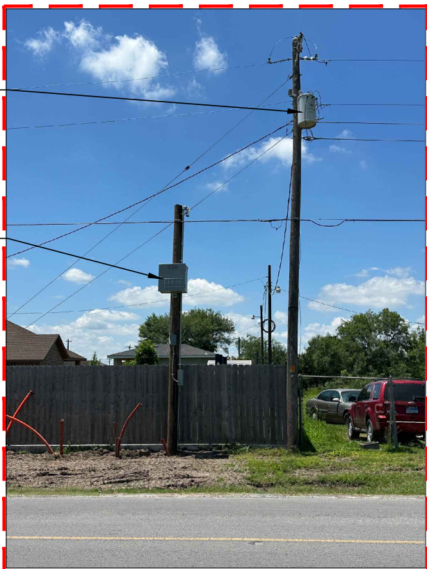
LAT: 26.275017° - LONG: -98.108196° NEW SPECTRUM POLE MOUNTED POWER SUPPLY 2' NORTH FROM ROW & 17' SOUTH FROM EOP
