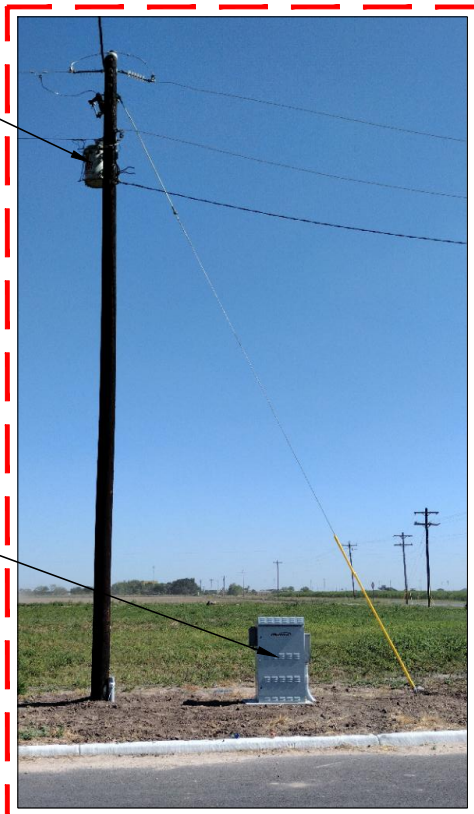
LAT: 26.309118° - LONG: -97.976990° NEW SPECTRUM UNDERGROUND POWER SUPPLY 3' NORTH FROM ROW & 6' SOUTH FROM EOP
