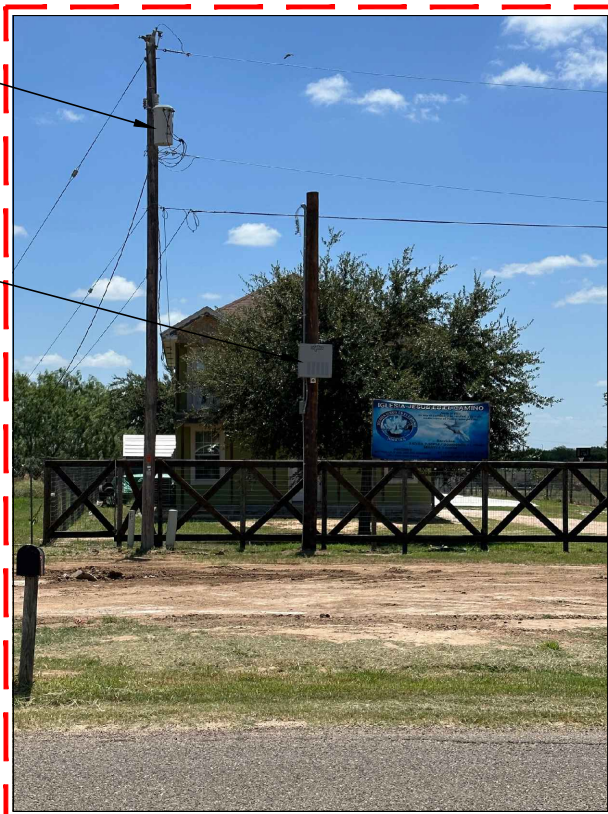
LAT: 26.385384° - LONG: -98.088409° NEW SPECTRUM POLE MOUNTED POWER SUPPLY 3' WEST FROM ROW & 54' EAST FROM EOP
