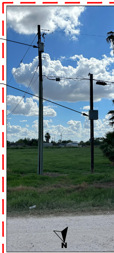
LAT: 26.290087° - LONG: -98.127685° NEW SPECTRUM POLE MOUNTED POWER SUPPLY 3' NORTH FROM ROW & 15' SOUTH FROM EOP
