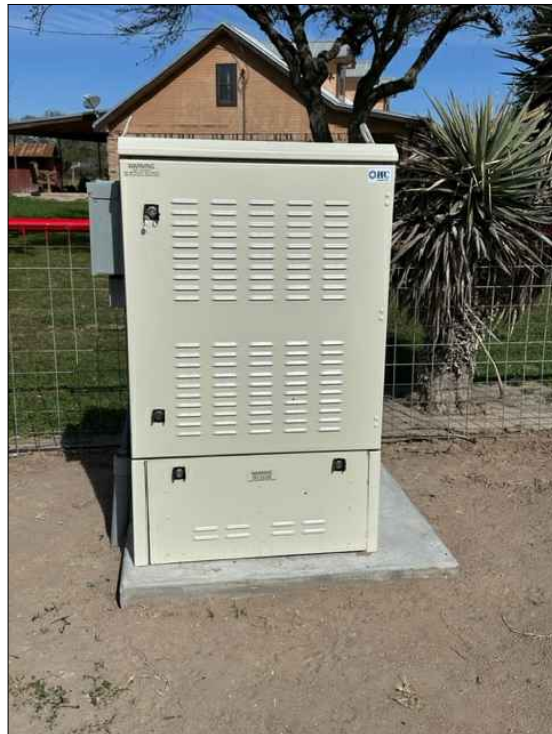
POWER SUPPLY UNIT / CABINET PICTURE-1 NOT TO SCALE
