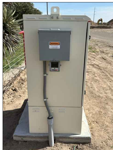
POWER SUPPLY UNIT / CABINET PICTURE-2 NOT TO SCALE
