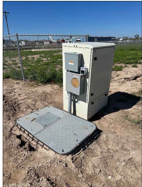
POWER SUPPLY UNIT / CABINET PICTURE-1 NOT TO SCALE
