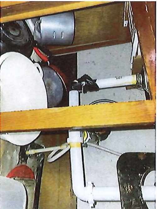
Mold and water damage in kitchen
