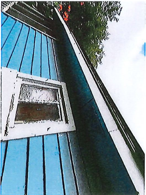
Siding inoperable windows and inoperable rear exit
