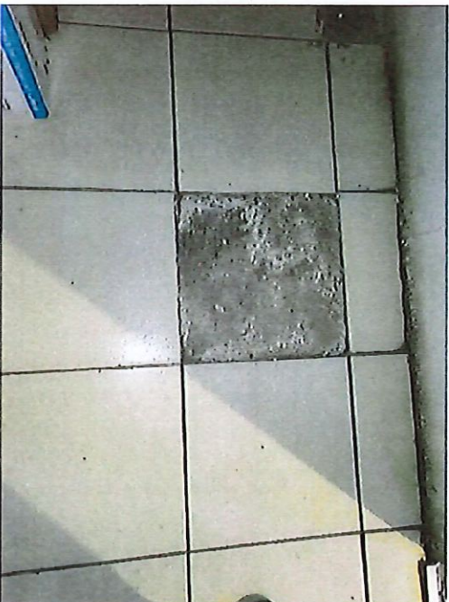
Missing & broken tiles
