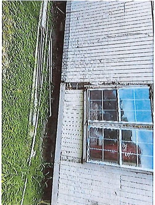
weather damaged Siding and inoperable windows
