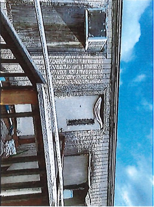
Back door inoperable and has big gaps
