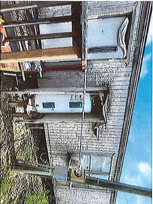
Water heater rusted and closet needs to be replaced
