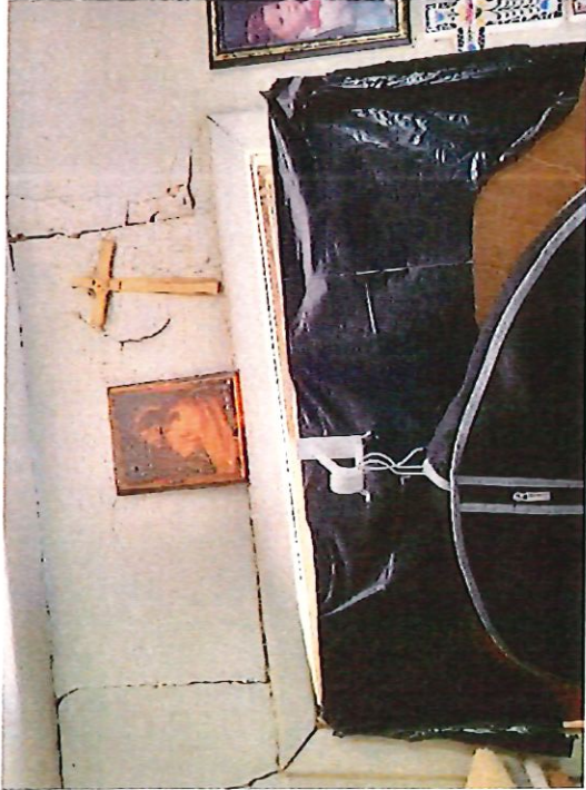
Exterior doors do not close properly.
