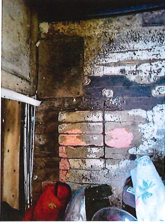
Subfloor exposed in 75% of the home
