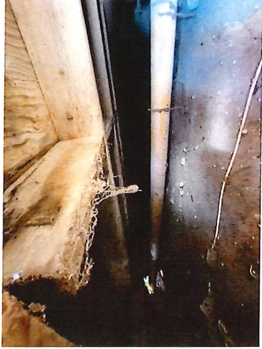
Sewer pipes not properly suspended or secured
