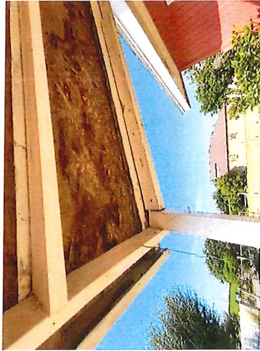
Front porch has mold and water damage
