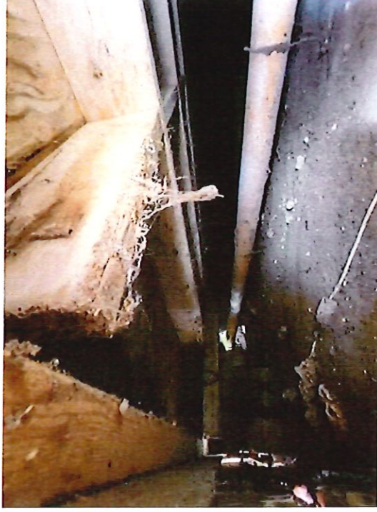
Sub-floor shows signs of water damage and rot
