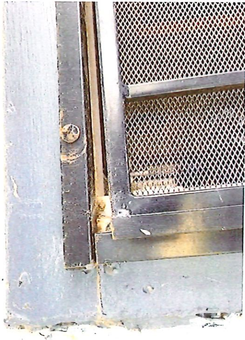
Exterior doors do not close properly.
