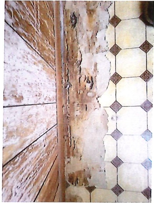
Sub-Floor shows signs of advanced termite Damage
