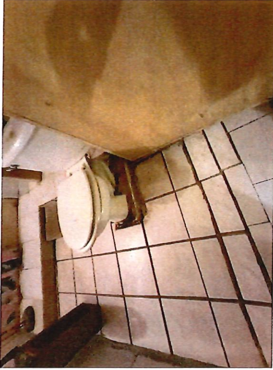
Raised uneven flooring
