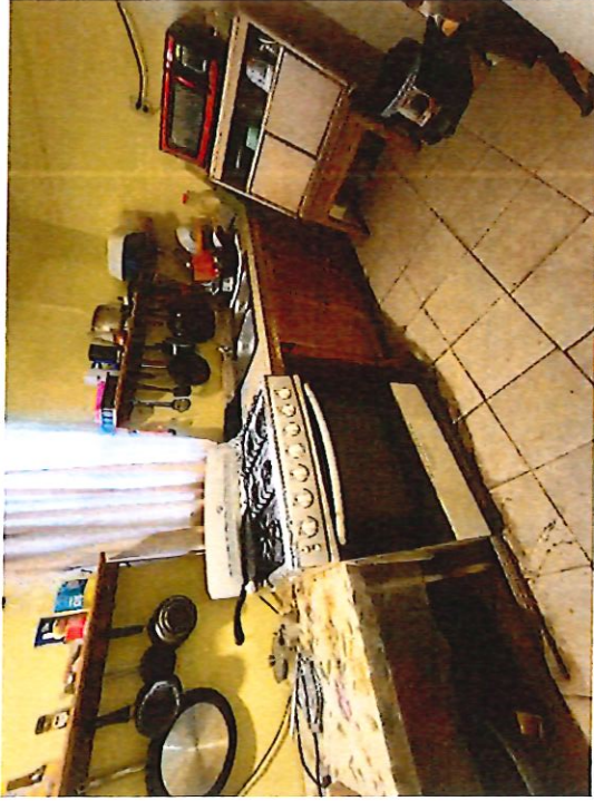
No cabinets and broken flooring
