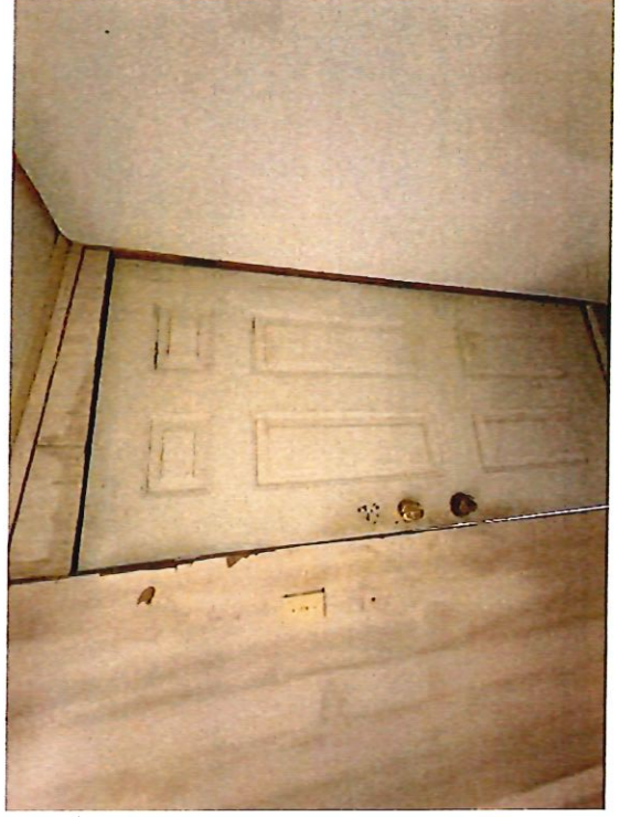
Exterior doors do not operate or seal properly
