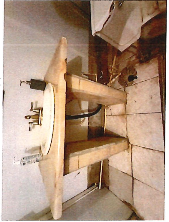
Make shift plumbing & Drain pipes
