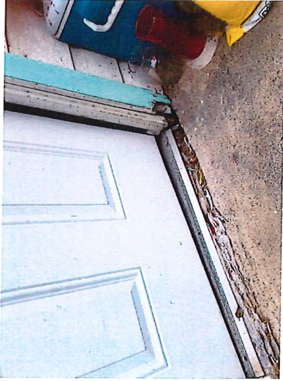
Exterior doors do not close properly.
