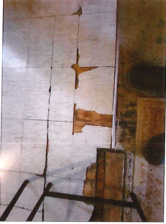
Subfloor exposed in 60% of the home
