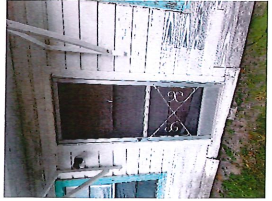
Steps need to be replaced
