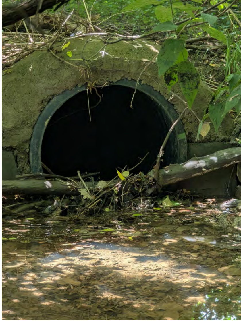
Culvert pipe outlet in the wooded area behind the property, partially obstructed by fallen branches and debris. Photographed July 12, 2026.
