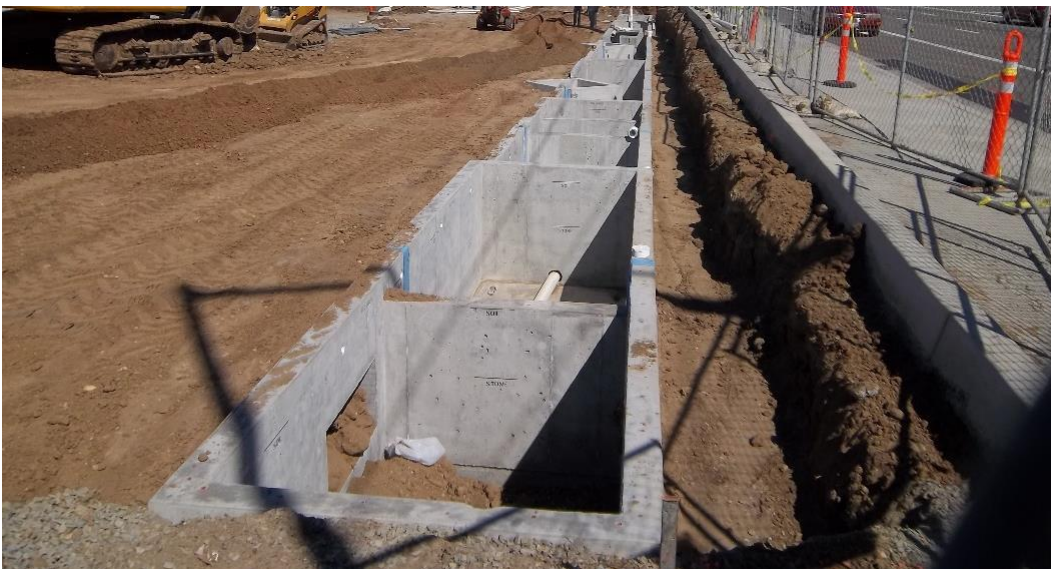
Stormwater detention basin installed as part of a commercial project to trap rainwater.
