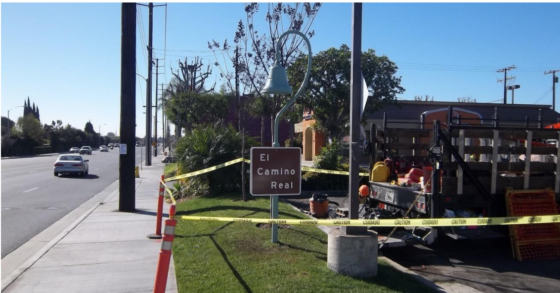
El Camino Real bell installed along the west side of Harbor Boulevard.
