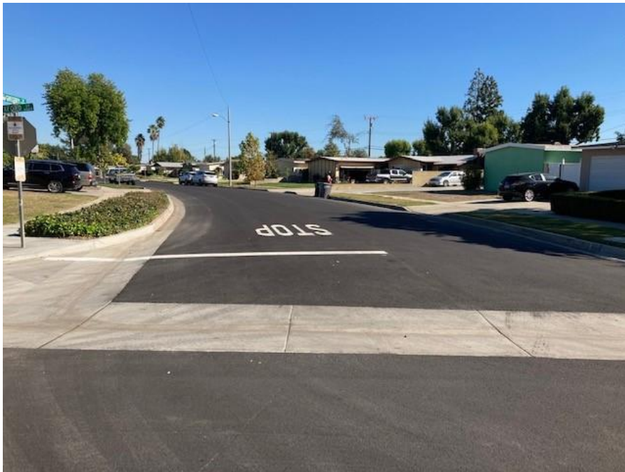
Gregory Ln at Dexford Dr – Final Concrete, Striping, Cross Gutter and Spandrels, facing East
