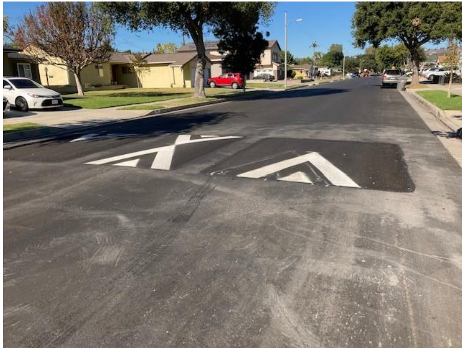
Painted Speed Lumps (typical)
