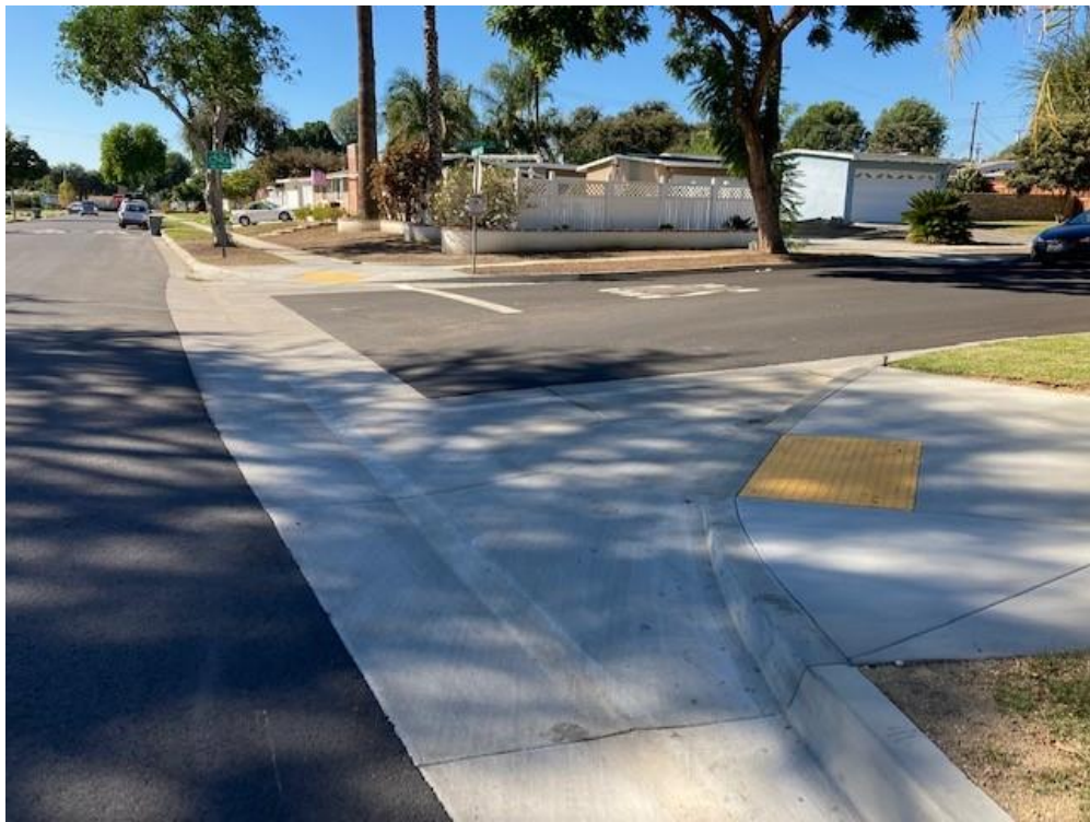
Gregory Ln and Chantry Dr – Completed Curb Ramp, Spandrel, Cross Gutter, Asphalt (Gregory Ln), and Slurry Seal (Chantry Dr)
