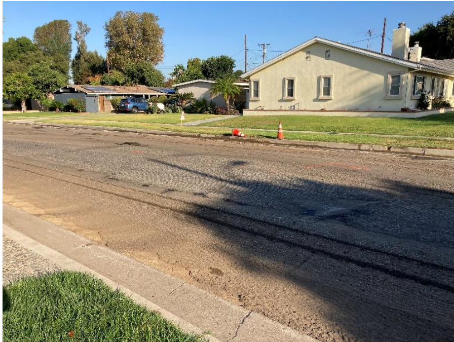
Gregory Ln – Milled Asphalt Surface, facing NW
