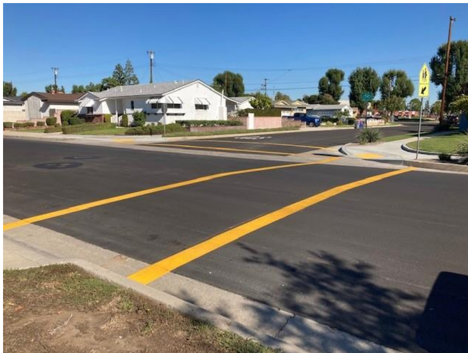
Dexford Dr and Morris Ave - Set-to-Grade Covers (typical) and Painted Crosswalks, facing NE
