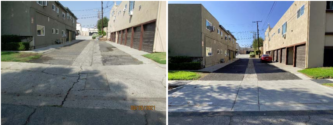
Alley improvement project showing before (left) and after (right), north of Stearns Avenue.
