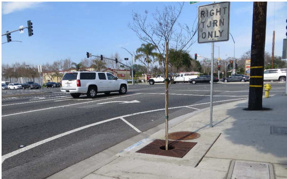
Stormwater “Filtera” unit with street tree used to filter rain water along the street (location: Beach Boulevard and Whittier Boulevard).
