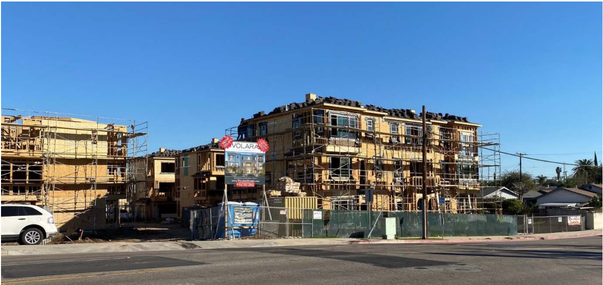
Volara residential project under construction at 104-118 East Electric Avenue which has a Development Agreement that was approved in 2020.
