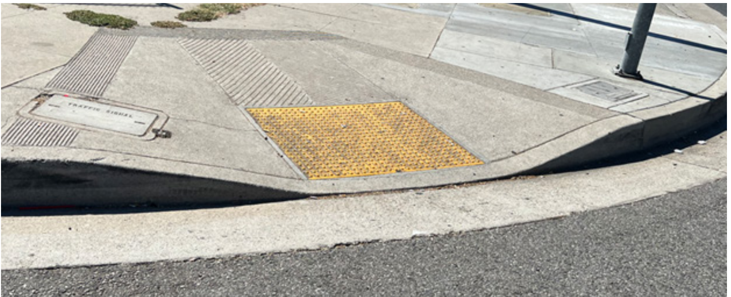
Harbor and Stearns – Ramp exceeds ADA maximum Slope
