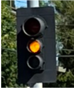
Substandard Signal Head
