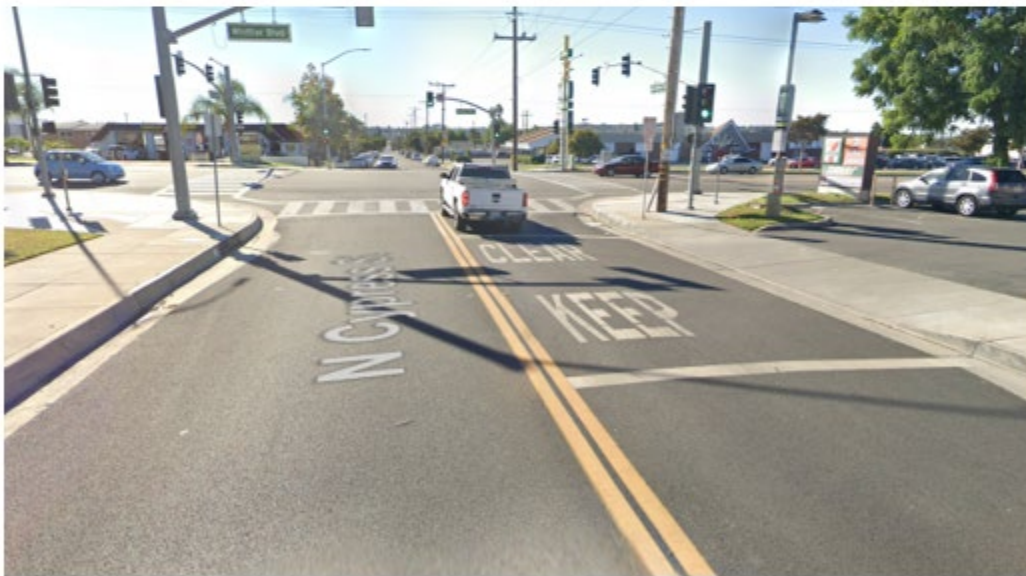
February 2023: Resurfacing of Cypress St. from La Habra Blvd. to S/O Bishop Drive
