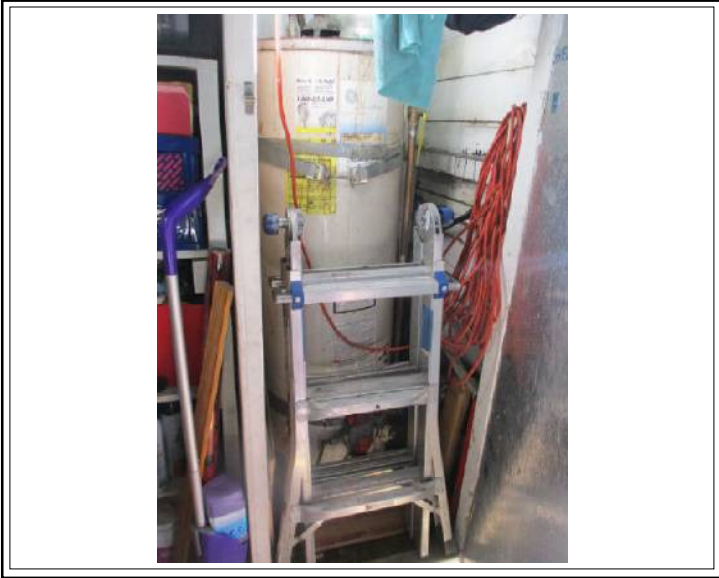
Water Heater - Unit 1
