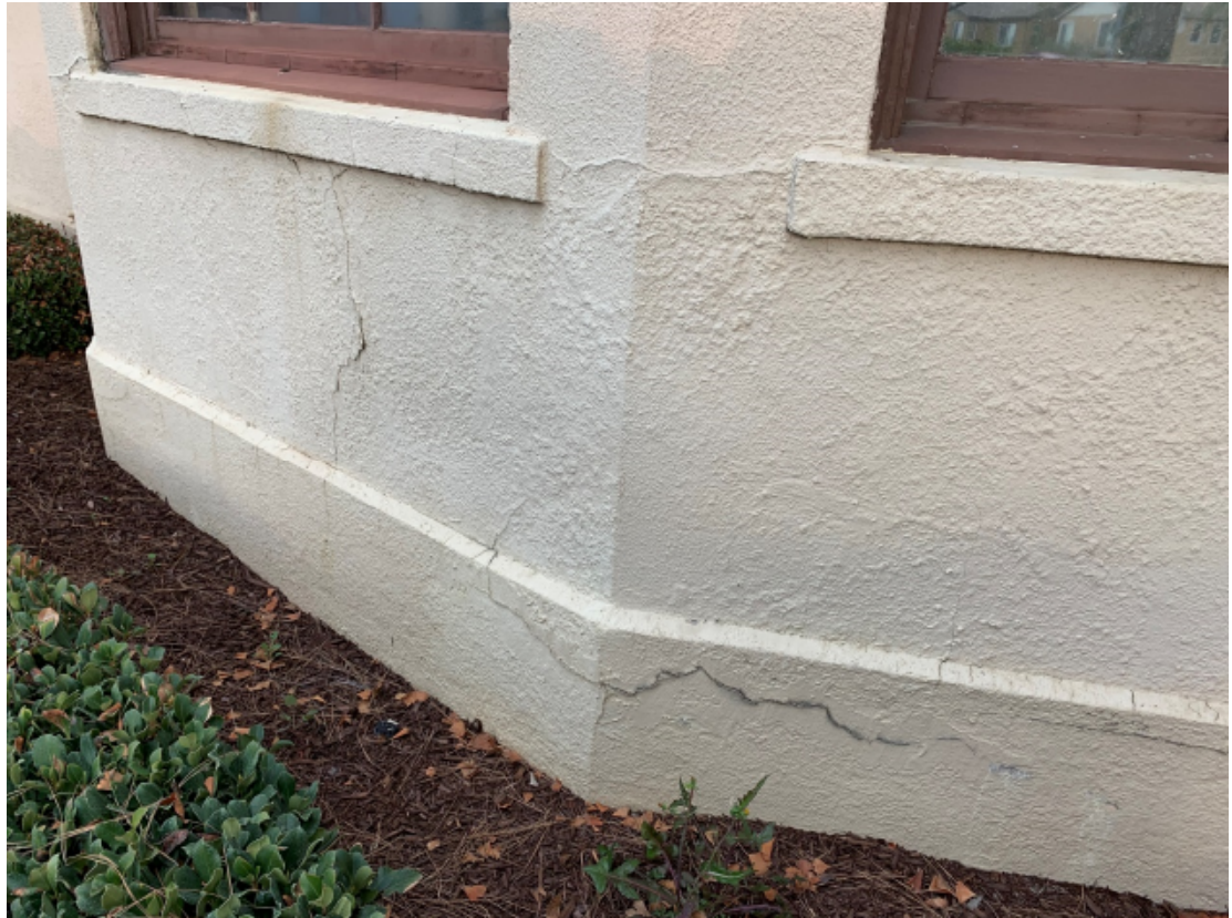
Photo 1 – Area A – Exterior Cracks in Finishes
