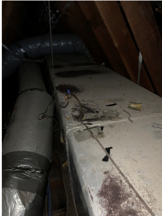
Photo 3 – Area A – Attic HVAC Duct. Notice termite fecal pellets on duct.
