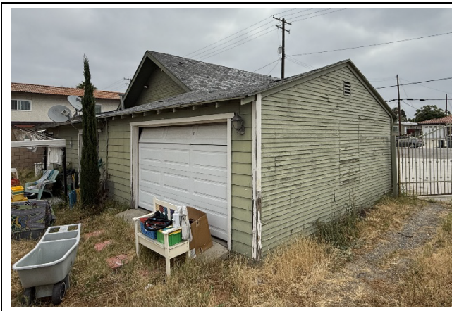
Image 3: Attached garage and rear addition, south elevation (right) and west elevation (left), view facing northeast. Source: GPA, June 2025.
