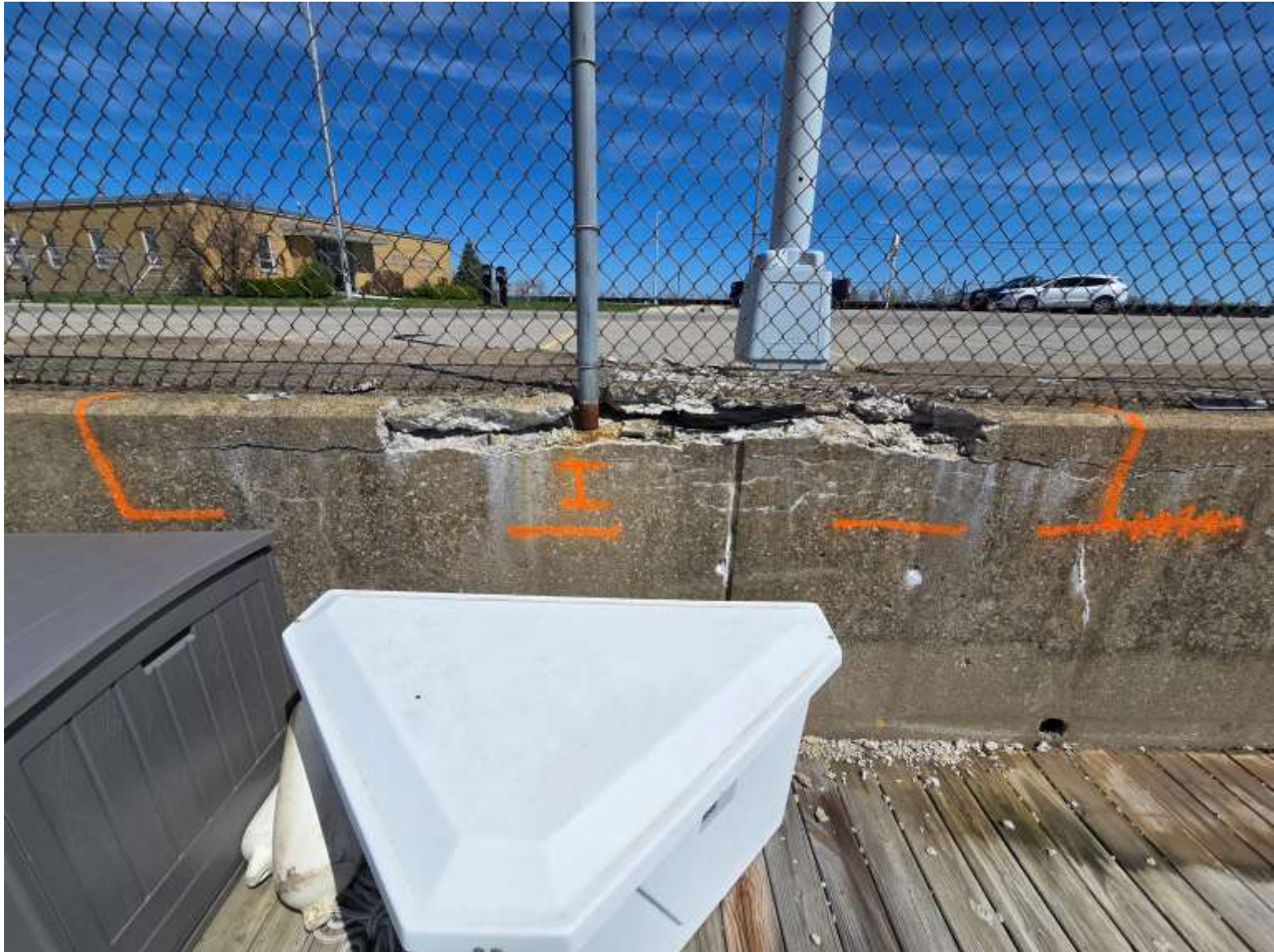
Lorain Engineering - Lorain Harbor Boat Club - patch I
