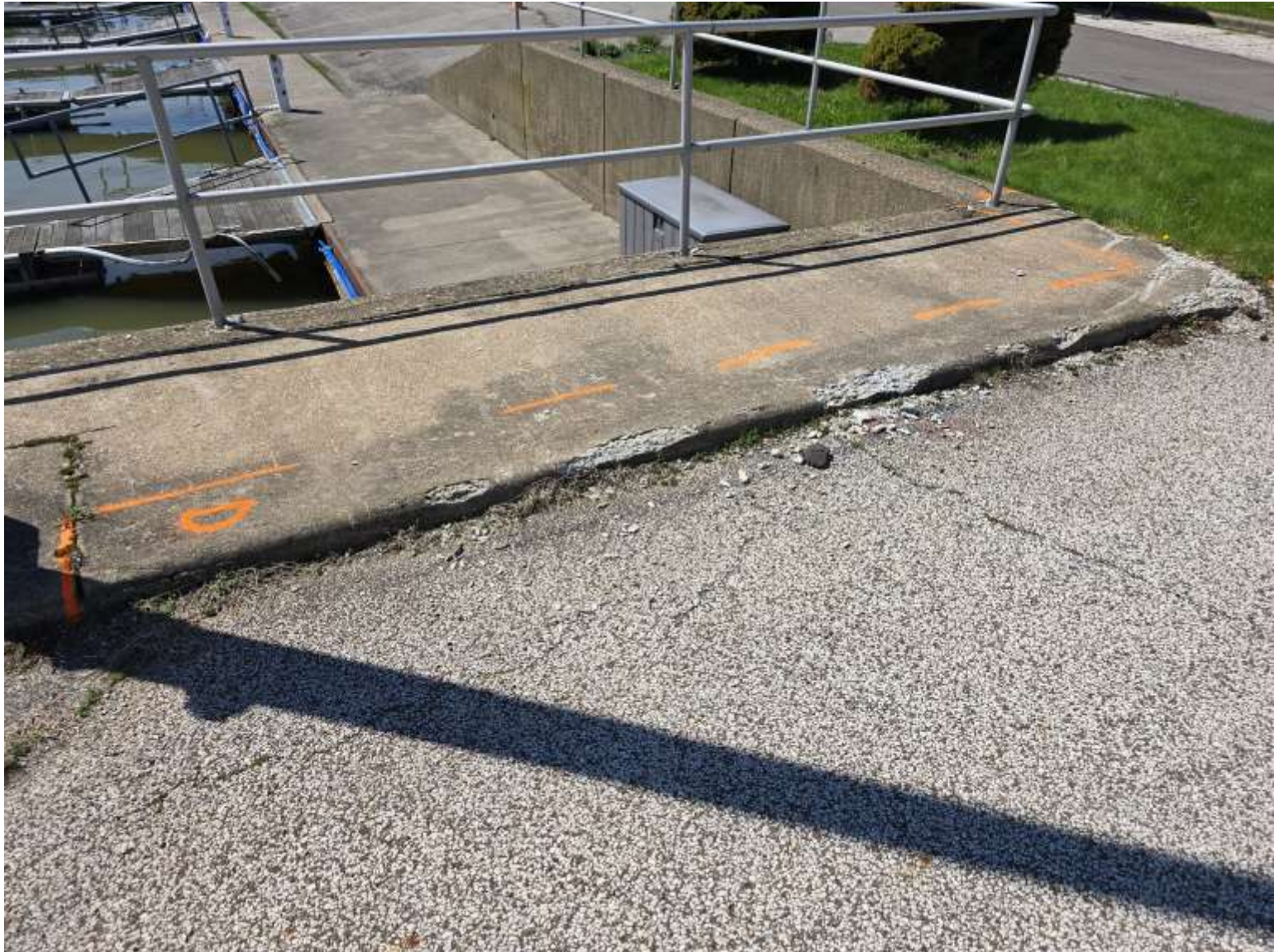
Lorain Engineering - Lorain Harbor Boat Club - patch D
