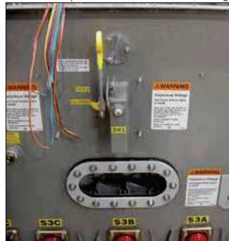
Figure 8. VFI transformer with visible break.
