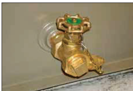
Figure 3. Drain valve with sampler.
