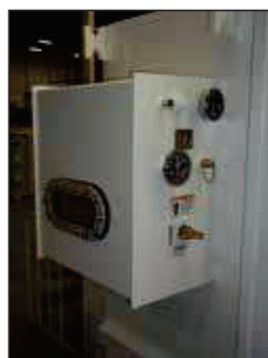
Figure 7. External visible break with gauges.
