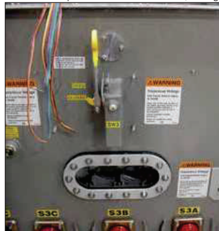
Figure 8. VFI transformer with visible break.
