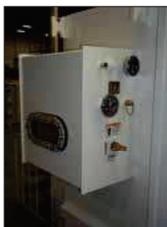
Figure 7. External visible break with gauges.
