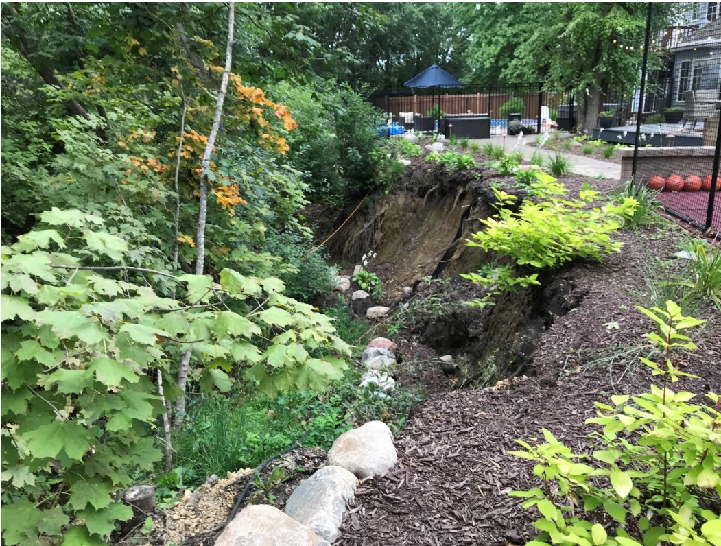
Figure 3. Slope Failure Head Scarp Looking West
