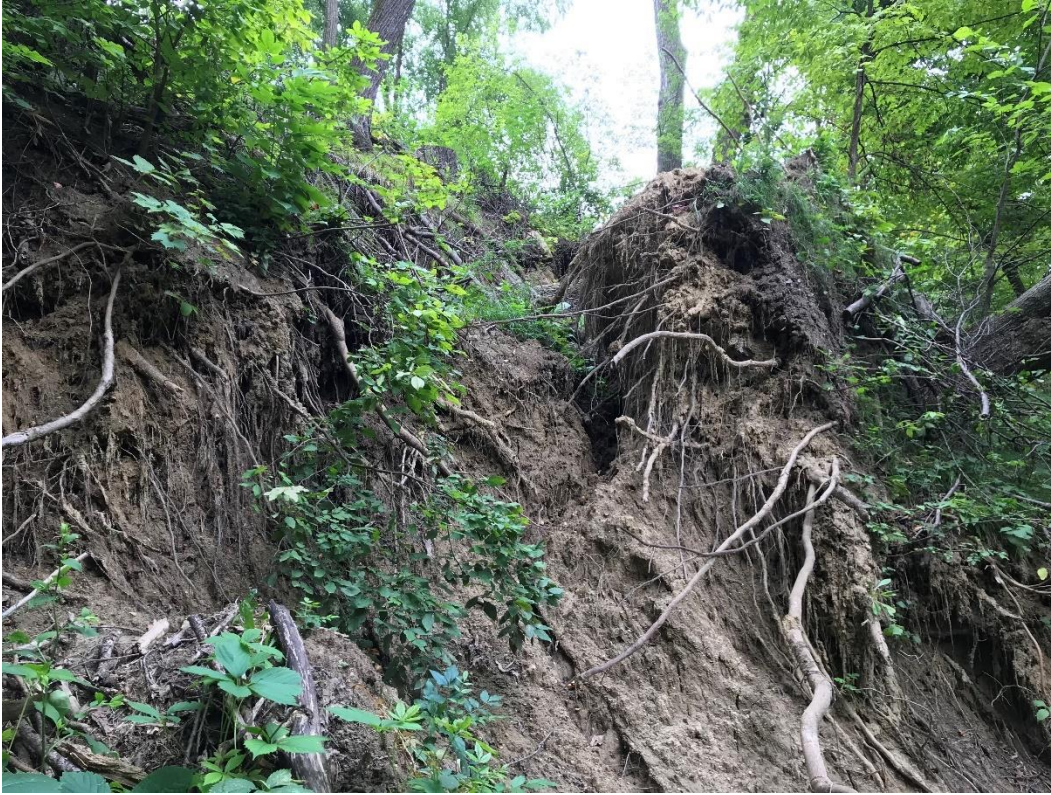
Figure 6. Lower Head Scarp Around Tree that Collapsed as Part of the Slope Failure
