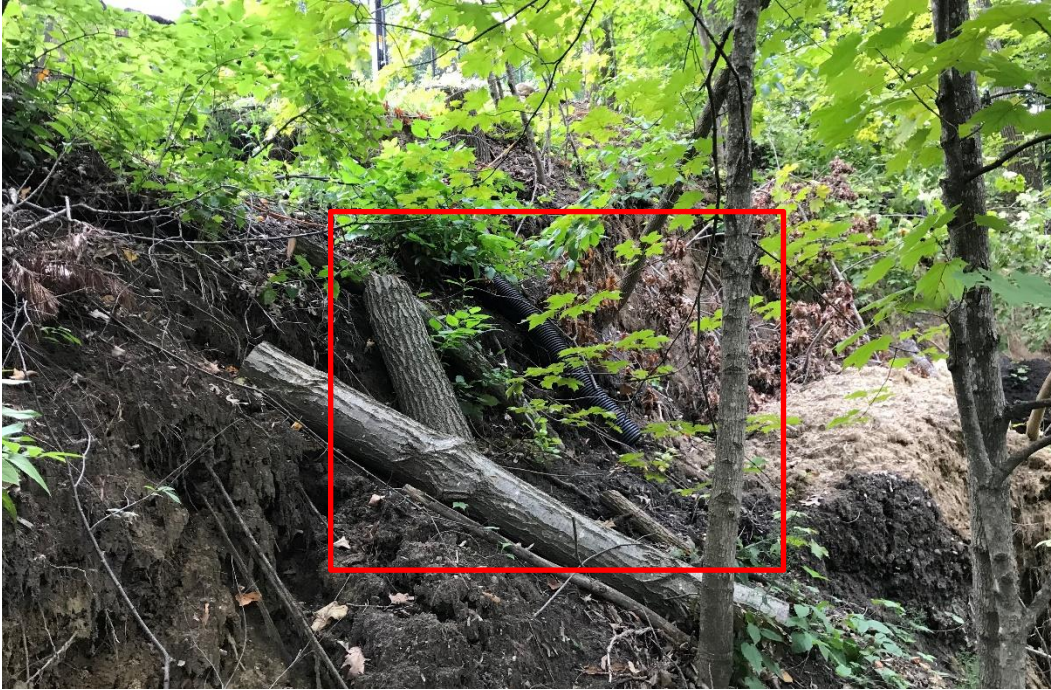
Figure 8. Drain Extending from House Partially Down the Slope Near Edge of Sport Court
