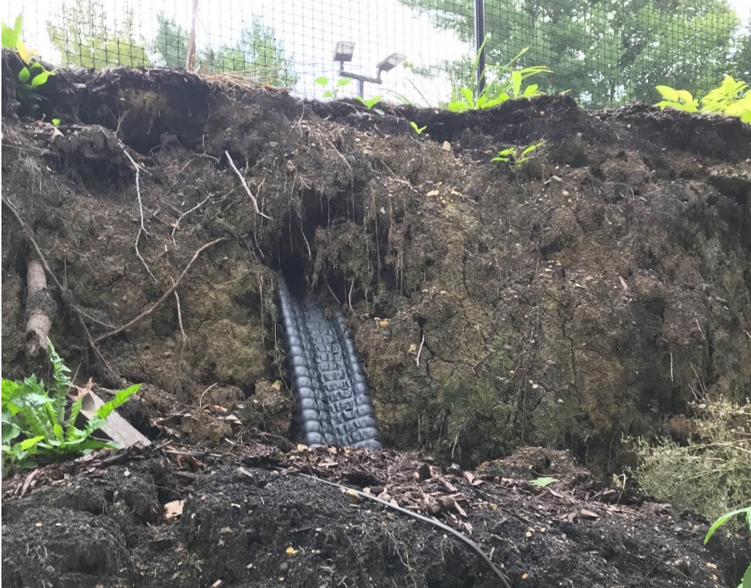
Figure 10. Buried Perforated Drain Extending into the Slope Near Edge of Sport Court
