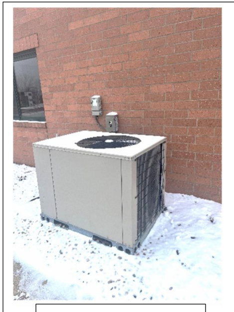
Outdoor AC Condenser
