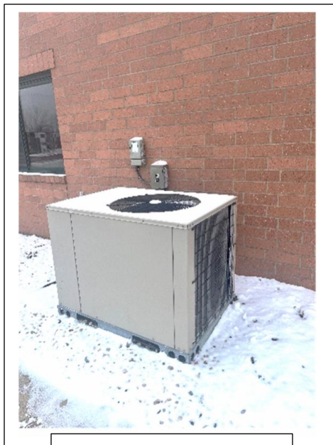
Outdoor AC Condenser
