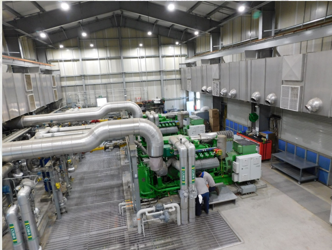
Existing Cogeneration Engines (with room for one more)
