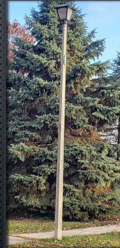
Cement pole w/coach fixture
