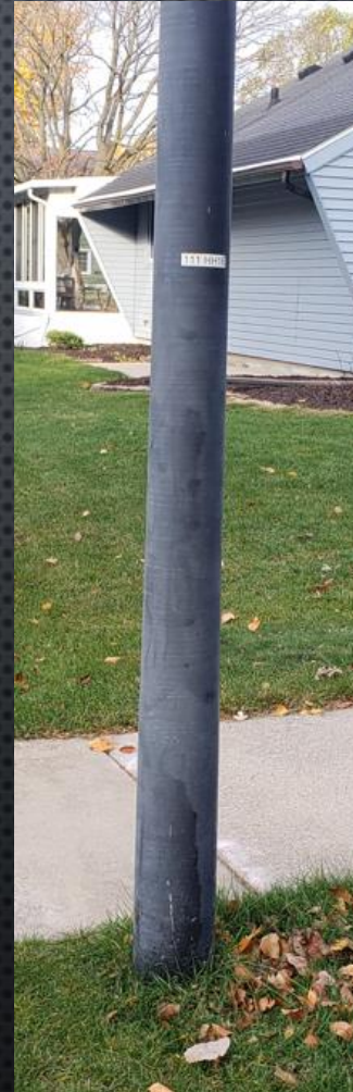
Current pole with deterioration
