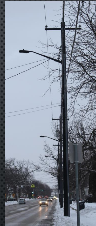
Fiberglass pole with cobra style fixture
