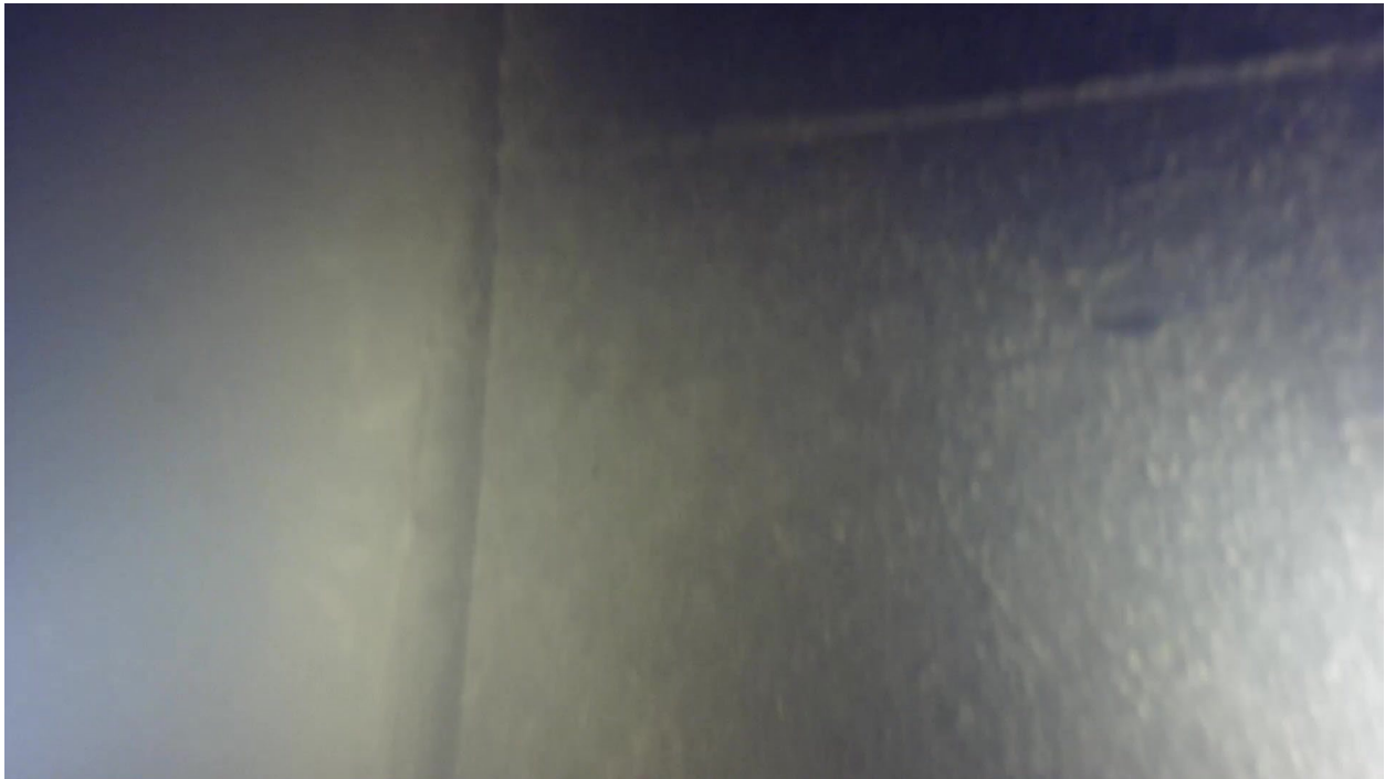
Figure 8 - Typical wall joint with offset greater near bottom of wall
