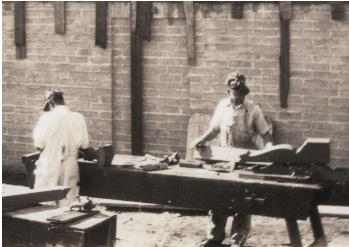
Skilled woodworkers preparing corbels for the living room beams on site ca. 1931. (Courtesy of Mary Kummings and Steve Scott)
