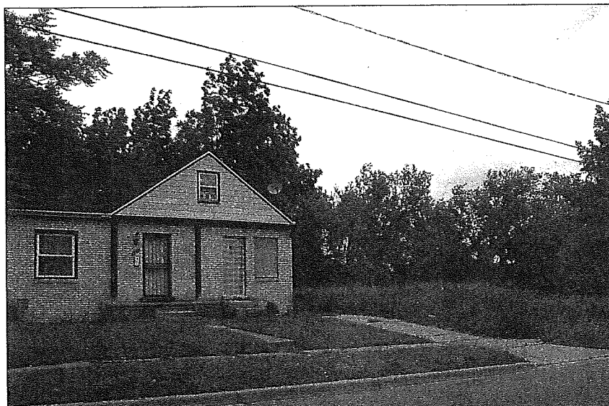
⊕ This partially boarded-up building in Flint, Michigan, sits next to a vacant lot overrun with vegetation.
