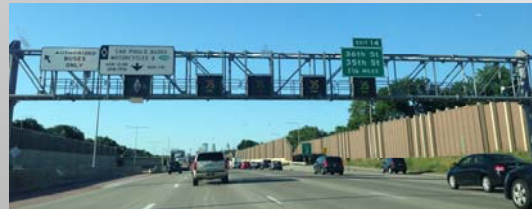
Overhead Lane Use Signs
