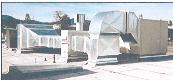
Roof Mounted HVAC and Exhaust System
