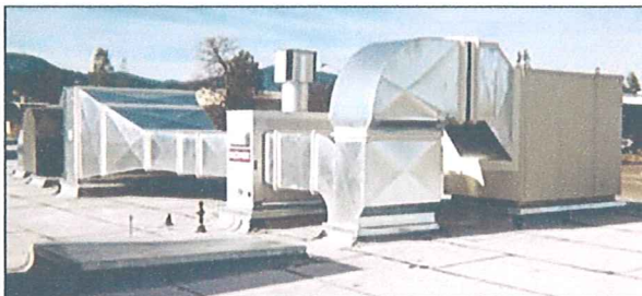
Roof Mounted HVAC and Exhaust System
