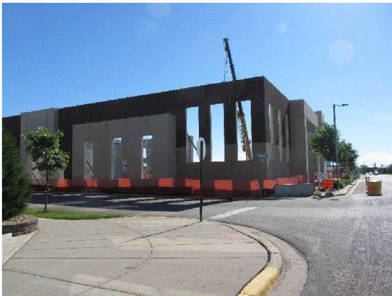
Photo taken June 27, 2013 at Sunwood Drive and Peridot Street looking north east.
