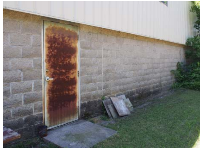
Figure B.I.9: Hollow metal door and frame rusting and signs of moisture damage at masonry wall along grade
