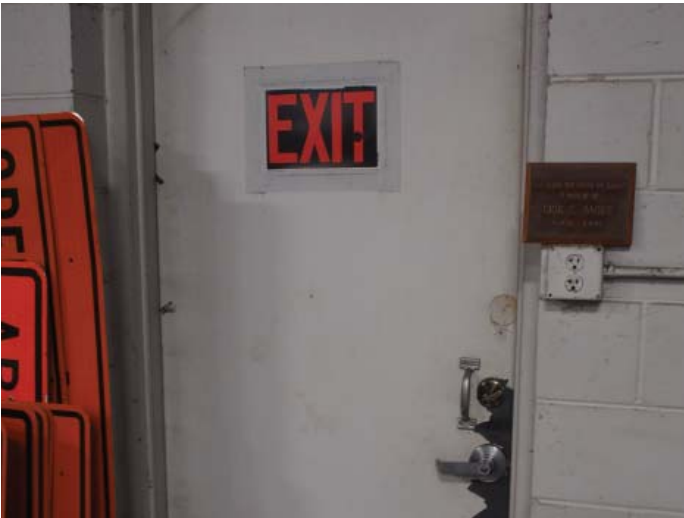
Figure B.I.12: Exit door has deadbolt with thumb-turn which is not allowed by code
