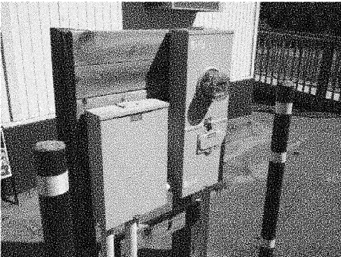
Figure B.5.12: Electrical systems are adequate and in good condition
