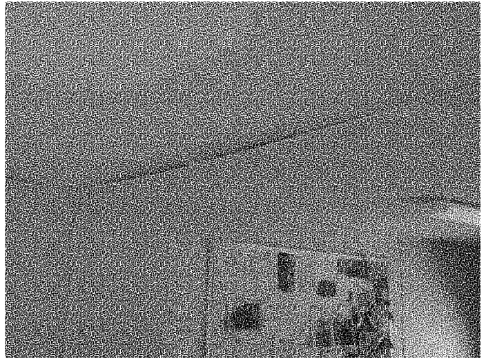
Figure B.5.3: Ceiling is starting to sag and separate at seam of trailer
