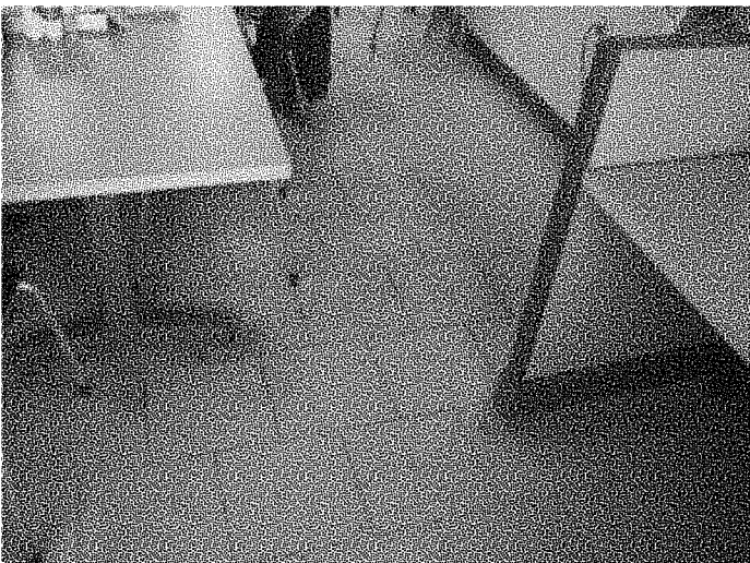
Figure B.5.7: VCT floor finish shows extensive wear
