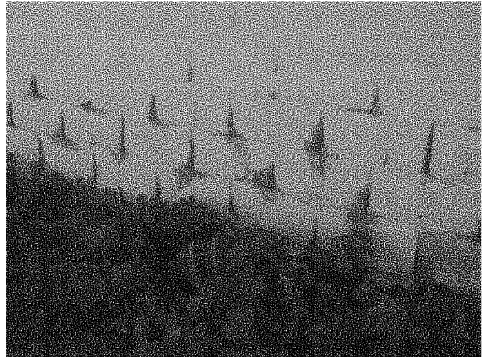
Figure B.3.8: Moisture damage is visible at base of masonry wall, exterior finish is failing and chipping off
