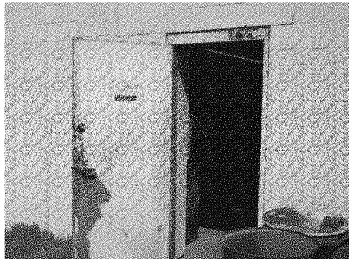
Figure B.3.3: Exterior hollow metal doors and frames are rusting
