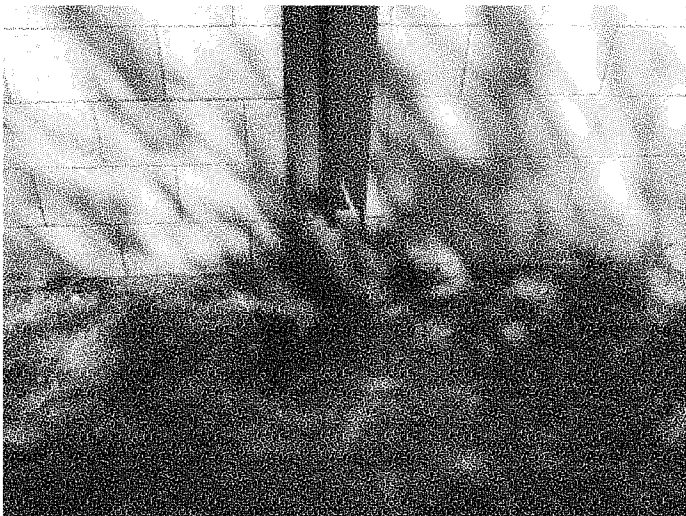
Figure B.3.7: Downspouts have eroded soil at base of wall/foundation causing potential drainage issues
