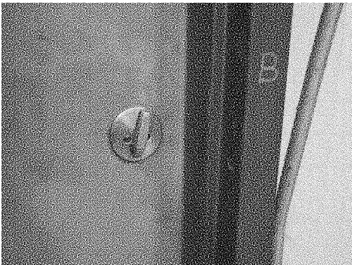
Figure B.2.7: Exit door is locked with deadbolt, does not meet code
