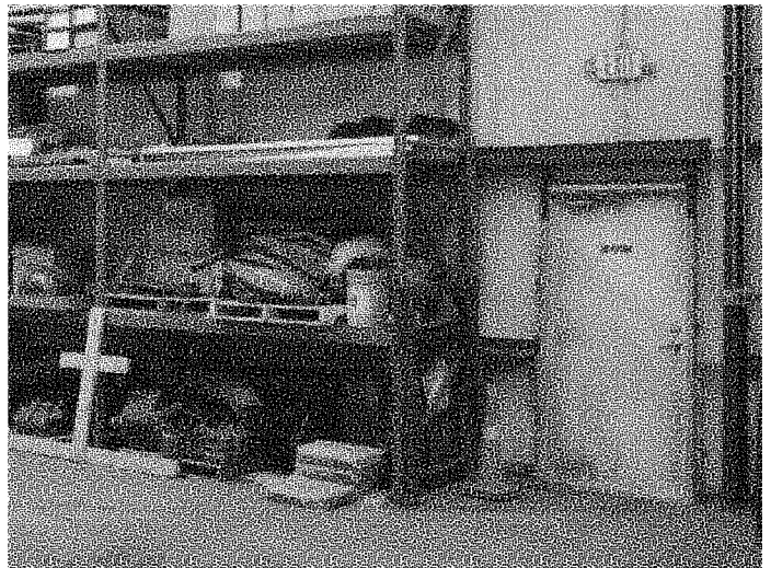
Figure B.2.3: Northwest exit door is stuck in closed position, does not meet code
