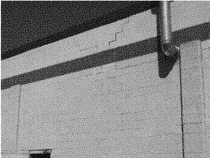
Figure B.3.5: Cracks are visible in exterior masonry walls on North and South facades
