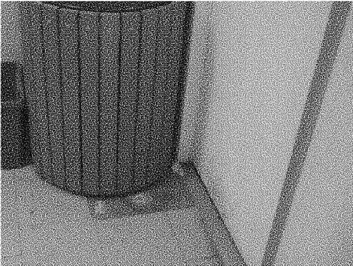
Figure B.5.5: Hole in floor is covered with sheet metal
