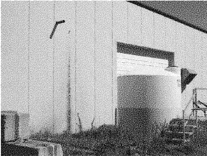
Figure B.2.5: Condensate drain is located high on the wall causing rust stains on South facade
