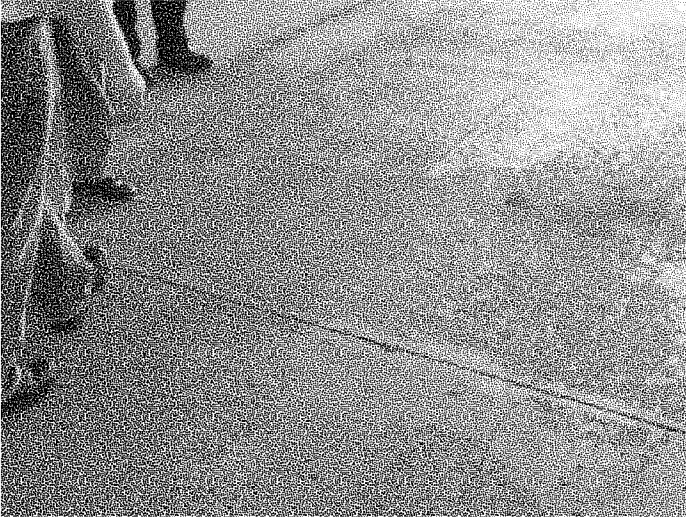
Figure B.3.11: Concrete slab on grade is heavily worn, spalling and cracking
