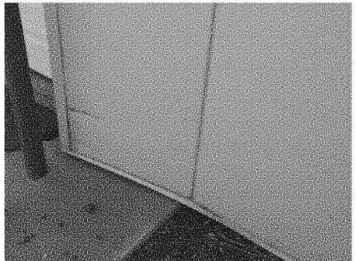
Figure B.2.10: Exterior metal panel cladding is damaged at North facade
