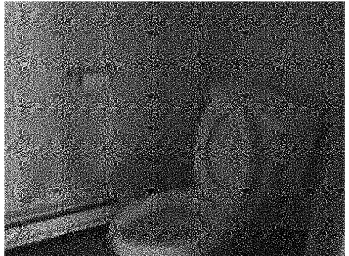
Figure B.1.15: Restroom is not handicap accessible
