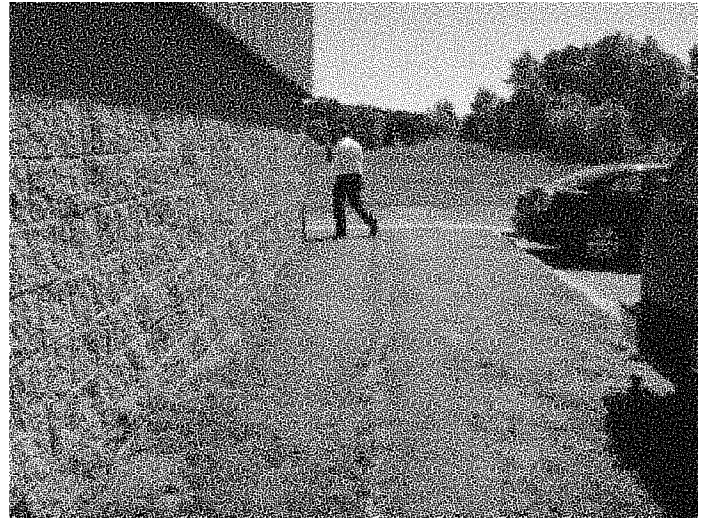
Figure B.I.8: Soil erosion at perimeter of building suggests evidence of gutters overflowing
