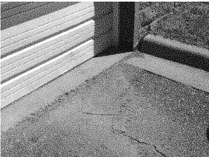
Figure B.I.7: Depressed asphalt at door threshold causing ponding and drainage issues
