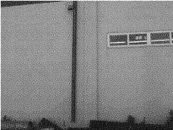
Figure B.3.6: Vertical cracks are visible in masonry pilaster at West facade
