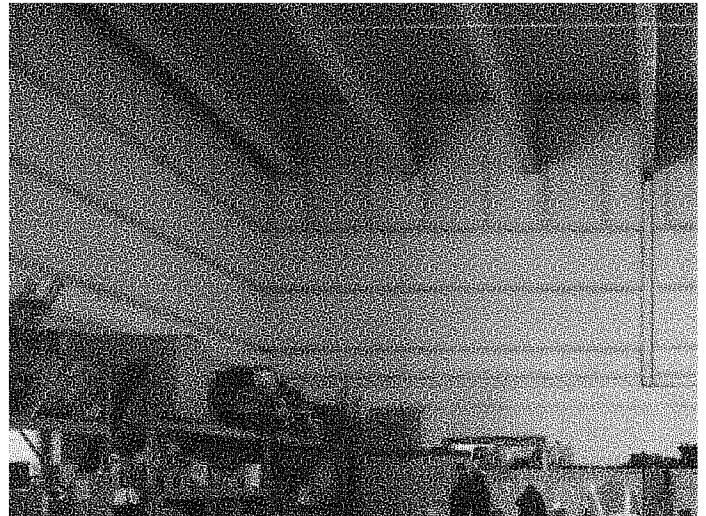
Figure B.3.9: Evidence of thermal bridging throughout the building as dirt has accumulated at areas of condensation aligning with the studs
