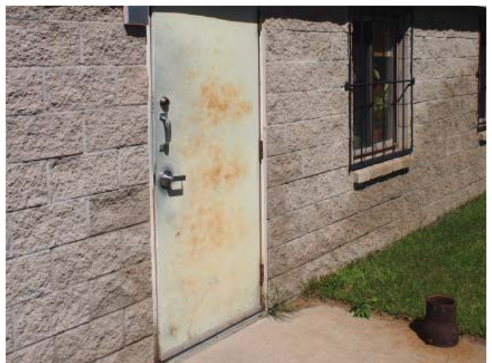
Figure B.I.10: Hollow metal door and frame rusting
