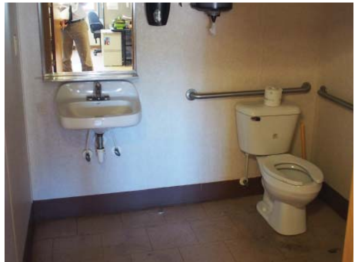
Figure B.5.10: Supply and waste pipes at lavatory are not insulated
