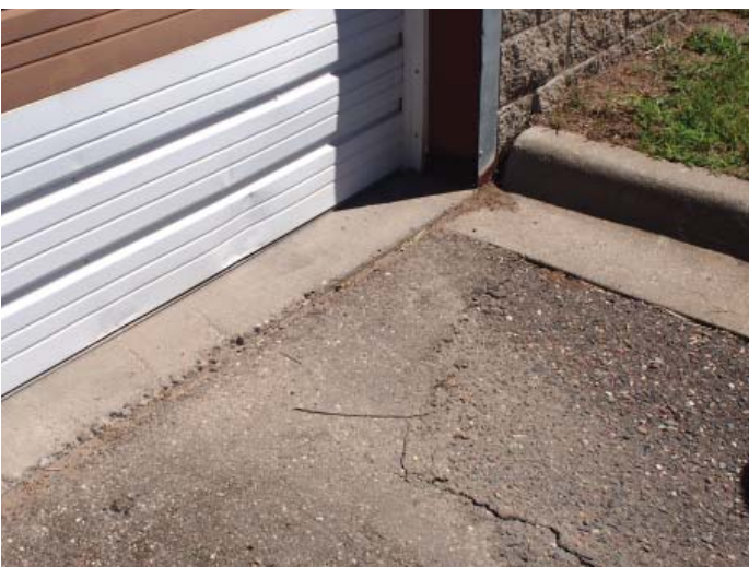
Figure B.I.7: Depressed asphalt at door threshold causing ponding and drainage issues
