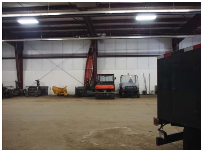
Figure B.2.4: Building lacks floor drains in main storage area creating slip hazards from wet vehicles
