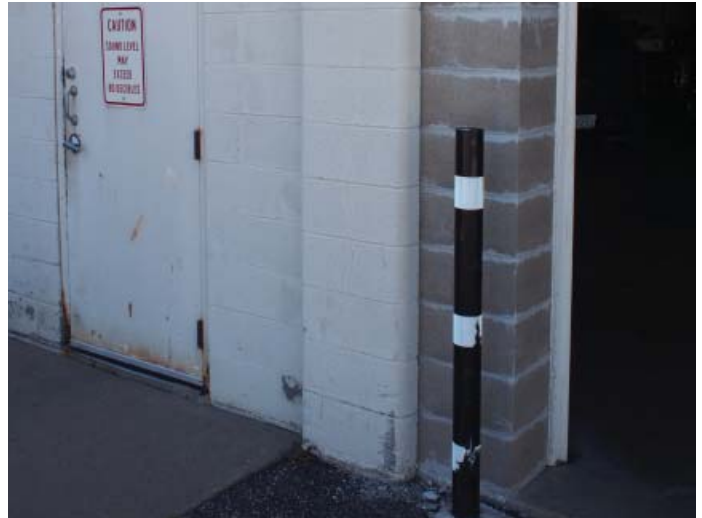
Figure B.3.2: Exterior masonry jambs have been repaired at overhead door but lack proper sealing/finishing
