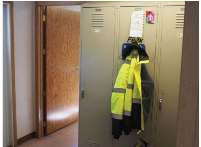
Figure B.5.9: Staff lockers are not handicap accessible
