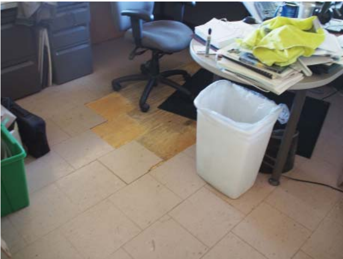
Figure B.5.6: Areas of missing VCT floor finish
