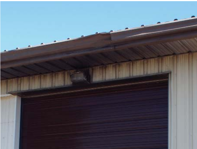
Figure B.I.6: Damaged metal gutter at overhead door
