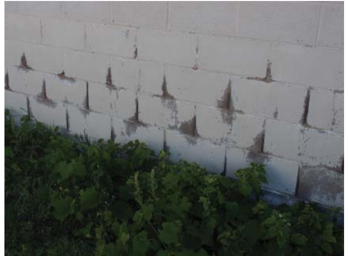
Figure B.3.8: Moisture damage is visible at base of masonry wall, exterior finish is failing and chipping off
