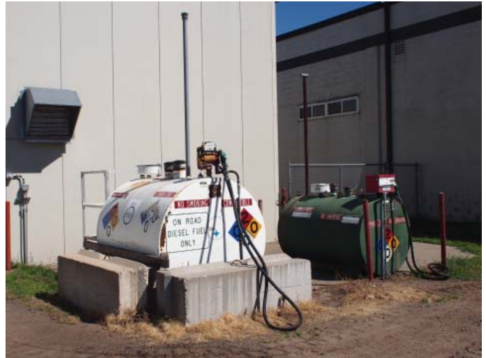
Figure B.7.1: Above ground fuel storage tank
