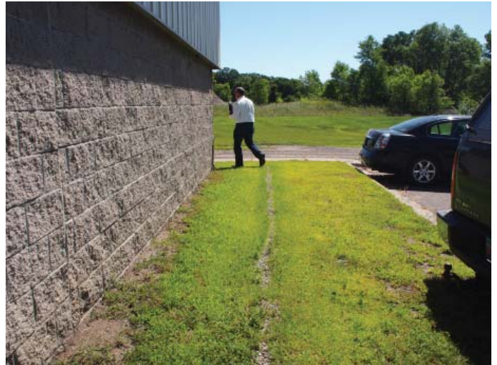
Figure B.I.8: Soil erosion at perimeter of building suggests evidence of gutters overflowing
