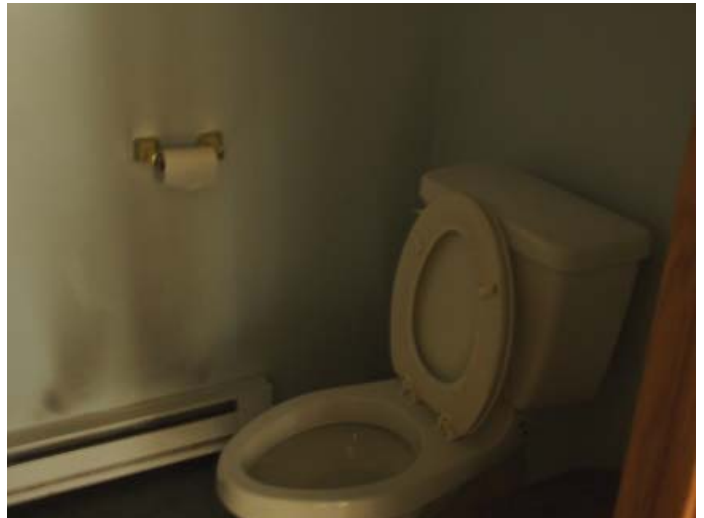
Figure B.1.15: Restroom is not handicap accessible
