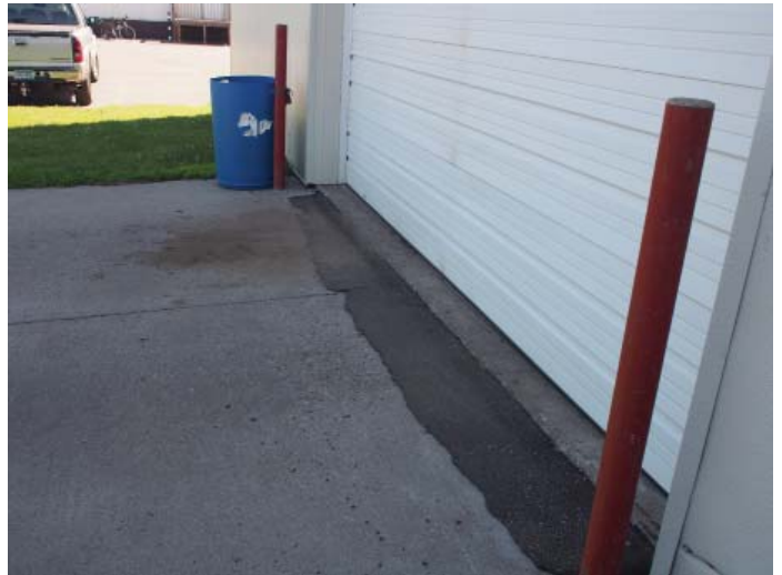
Figure B.2.9: Settling of concrete apron at North overhead door has necessitated asphalt patching
