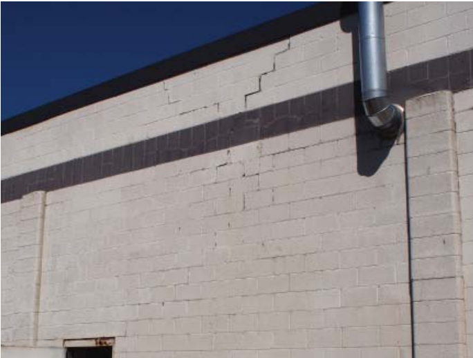
Figure B.3.5: Cracks are visible in exterior masonry walls on North and South facades
